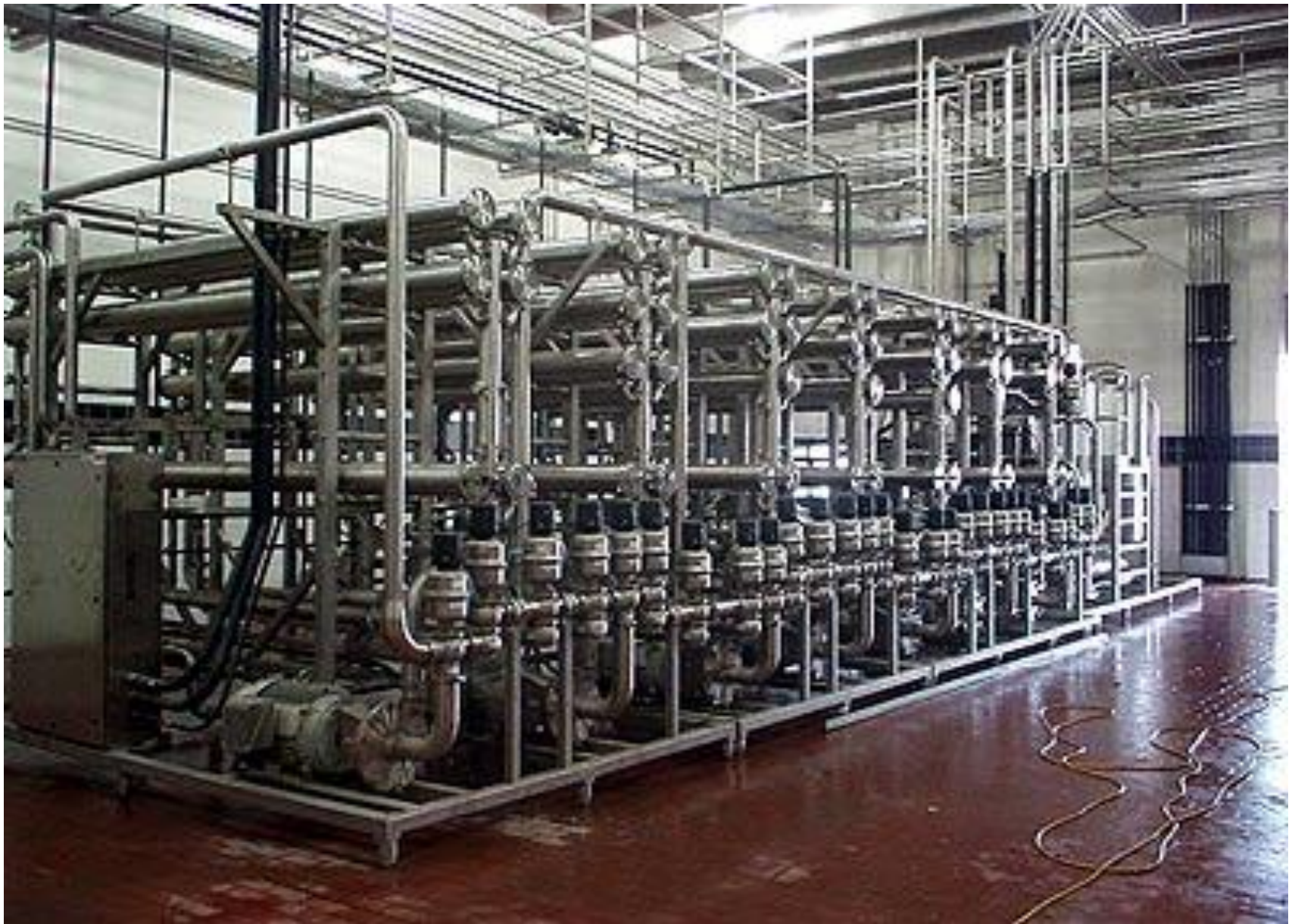
Large membrane filtration installation for whey processing.
