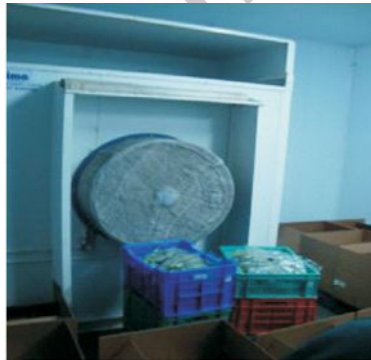
Fig. 10.2. Forced air cooling (High humidifier)
