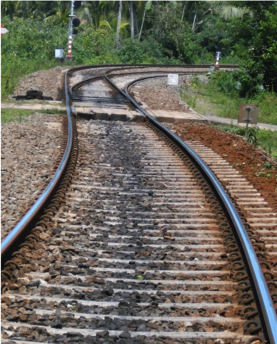
Left-Curve combined with a right-Hand-Turnout without a Transition; with a Change of the Gradient on the right diverging Route. Gintota, Sri Lanka, after the IRCON Upgrade
