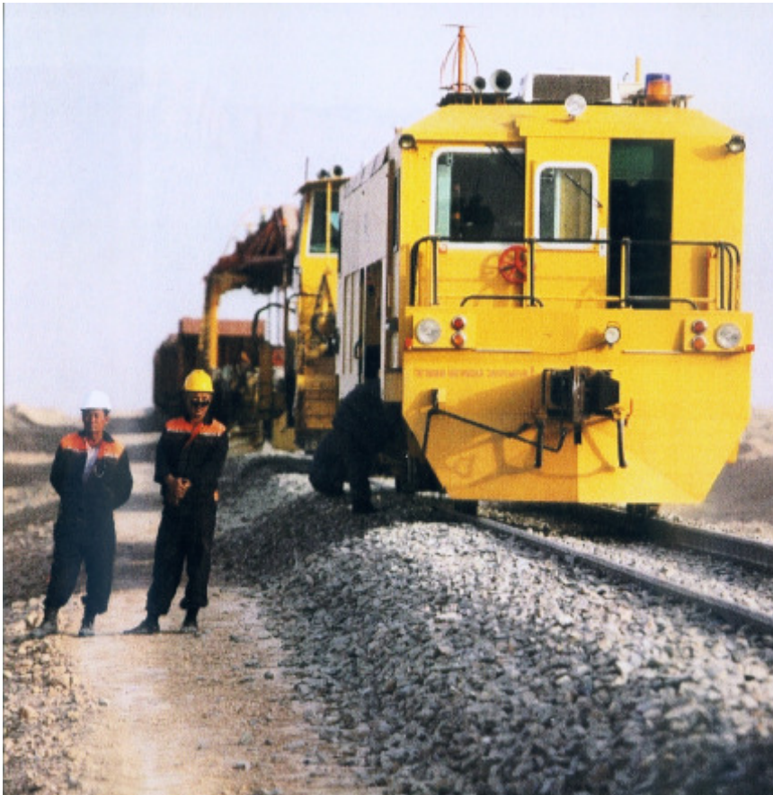
Machine Track-Tamping of a well profiled Track with Border Foot Path in North Afghanistan
