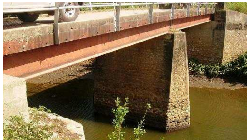
Wearing of Bridge pier due to the effect of running water
