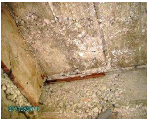
Poor formwork produces poor Workmanship
