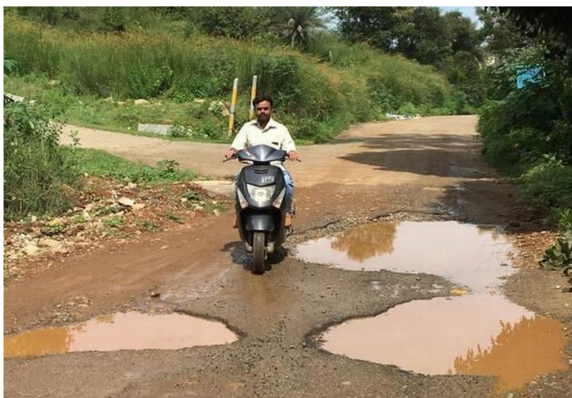
FIG.7 PATCHES ON ROAD WHICH LEAD ACCIDENTS
