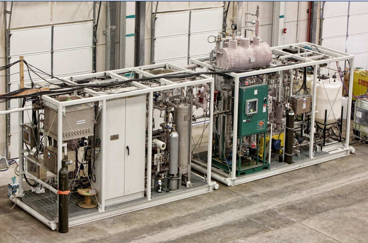
Designed, built, and commissioned by Merrick
