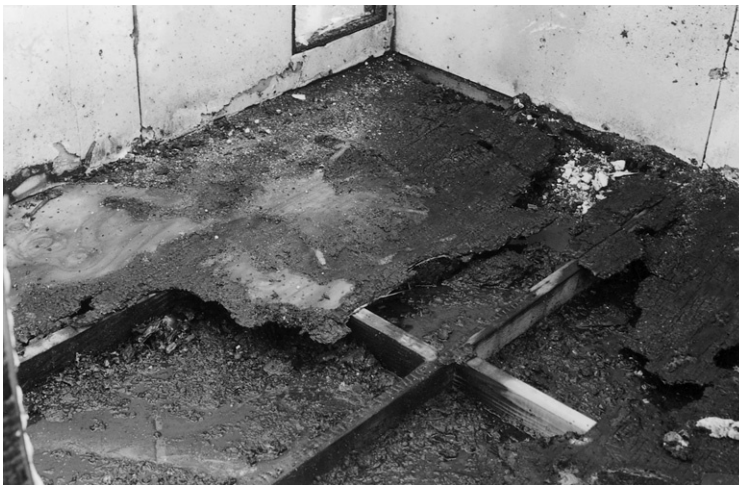
FIGURE 15.18 The exposed carpet and 1/2-inch plywood floor of this test cubicle were consumed by exposure to a postflashover fire of duration of less than 6 minutes.
