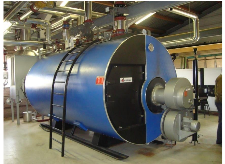
Centralized heating system
