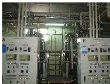
Control panel for the plant
