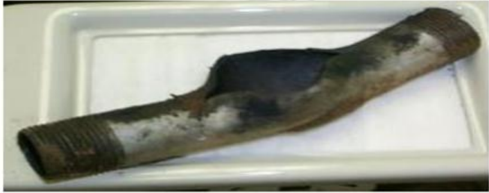
Soot marks and its deposition
