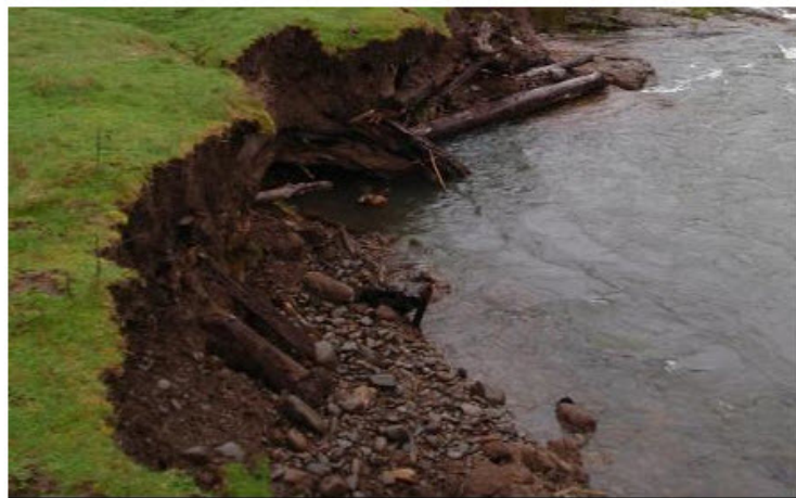
Fig. 3.5. Stream bank erosion. (Source: www.sswc.org )
