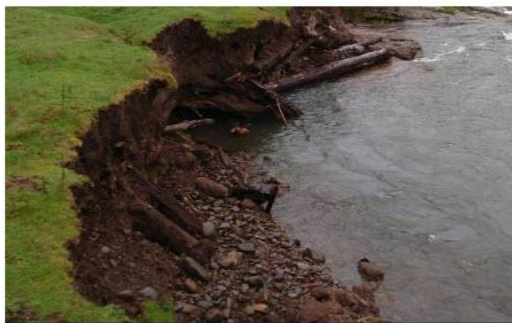
Fig. 3.5. Stream bank erosion.
